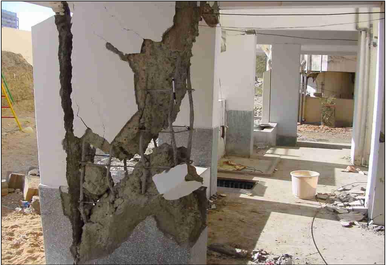
Figure 6: 230 mm wide columns in ground storey of RC Frame Buildings: damaged column in Bhuj town during 2001 Bhuj earthquake
